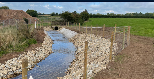
2021: A project delivered for Cadent Gas to carry out improvement works to cover and protect a vulnerable section of a high-pressure pipeline.
