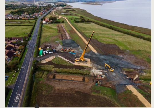
2021: Our flood protection scheme at South Ferriby received an ‘Environmental Best Practice’ Green Apple Award, recognised as a low carbon environmental project.
